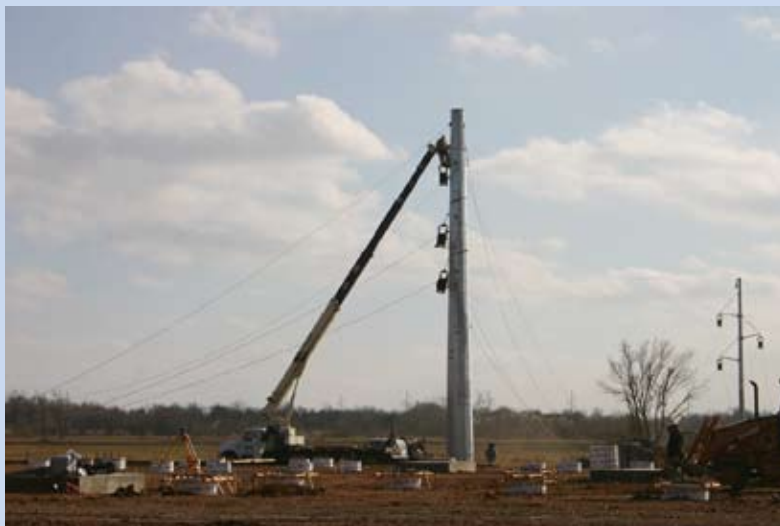
Construction of the new transmission line, running from GRDA's Coal Fired Complex to a new substation near the Google facility will help improve reliability in the MidAmerica Industrial Park.
