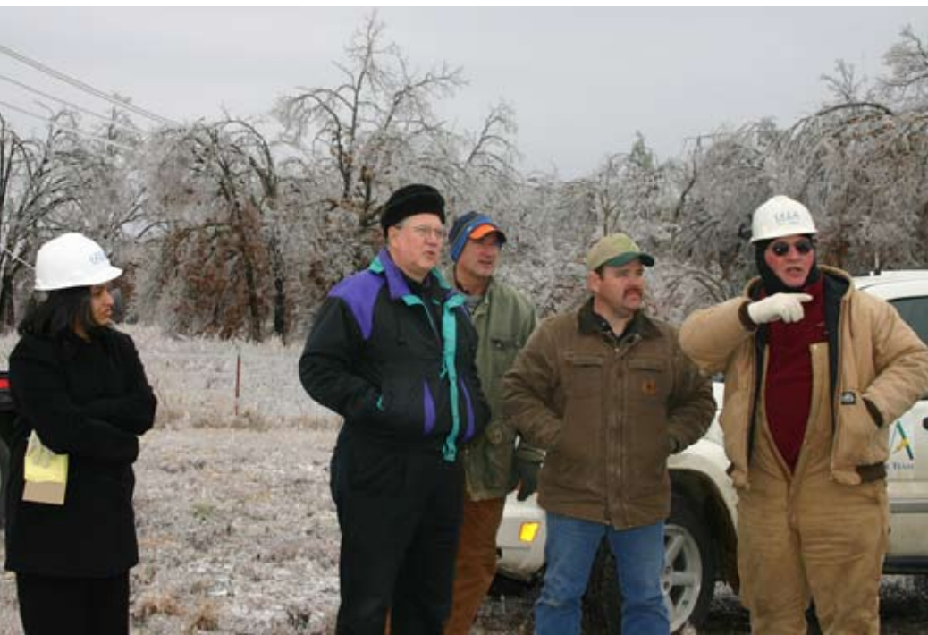
Left: (From l to r) GRDA's Nishi Ninan, Bud Averill, Phil Stoke, Mike Harris and Jerry Johnson survey the damage to the 412 Substation following January 2007's ice storm.
