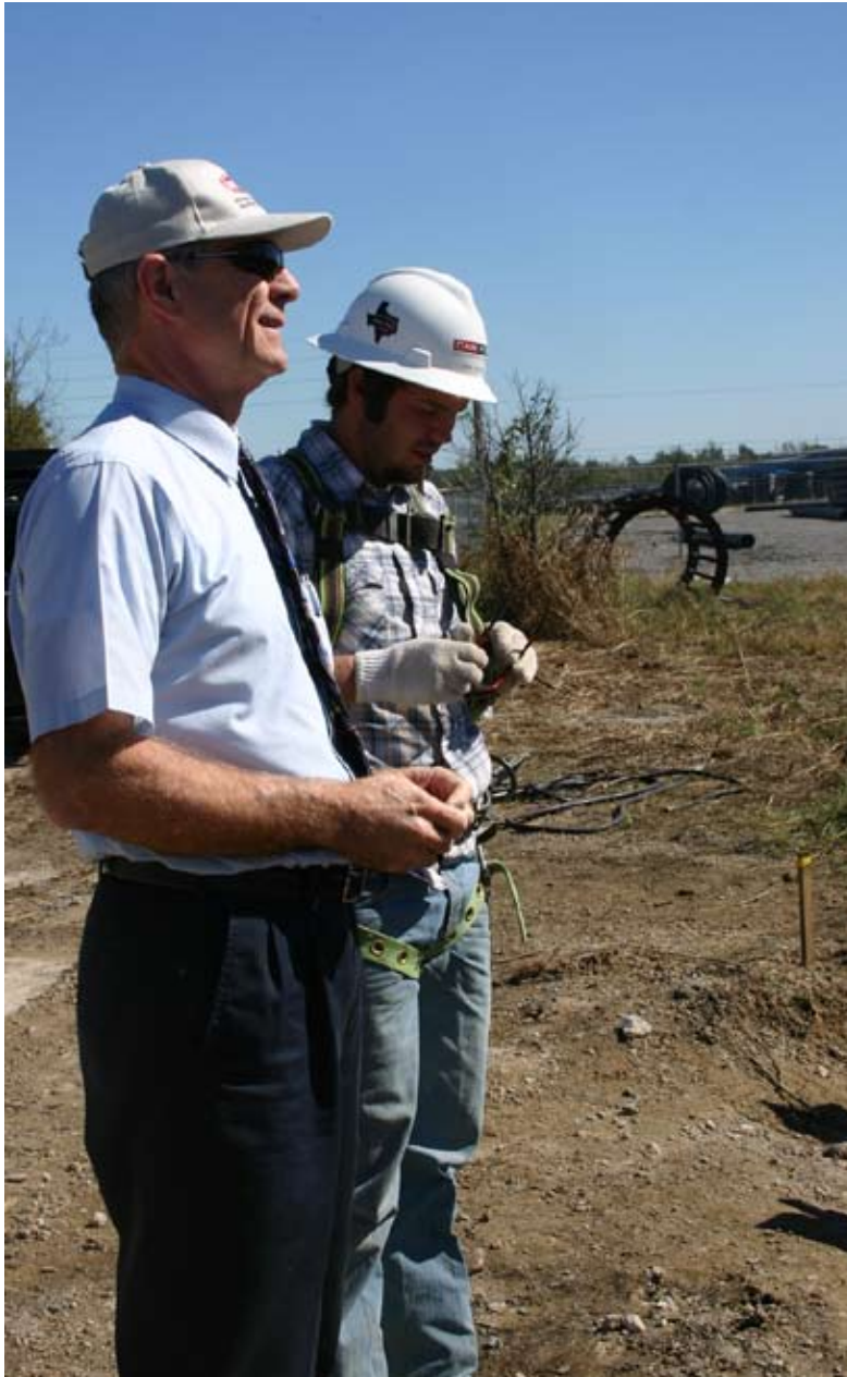
Mike Herron, GRDA Chief Engineer (left) with contractor from CanFer at a dead end tower foundation site on the MAID 161 kV transmission line.
