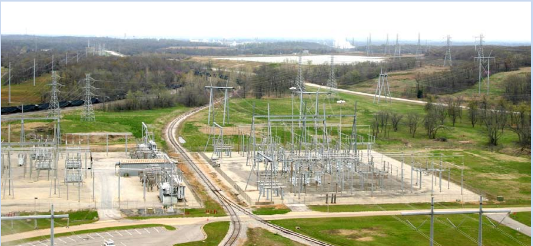
NEXT DOOR NEIGHBOR ... Looking north, from the Unit 2 boiler at the GRDA Coal Fired Complex. The industries of the MidAmerica Industrial Park can be seen in the distance. High voltage transmission lines (both sides of the picture) help insure reliability to those industries.
