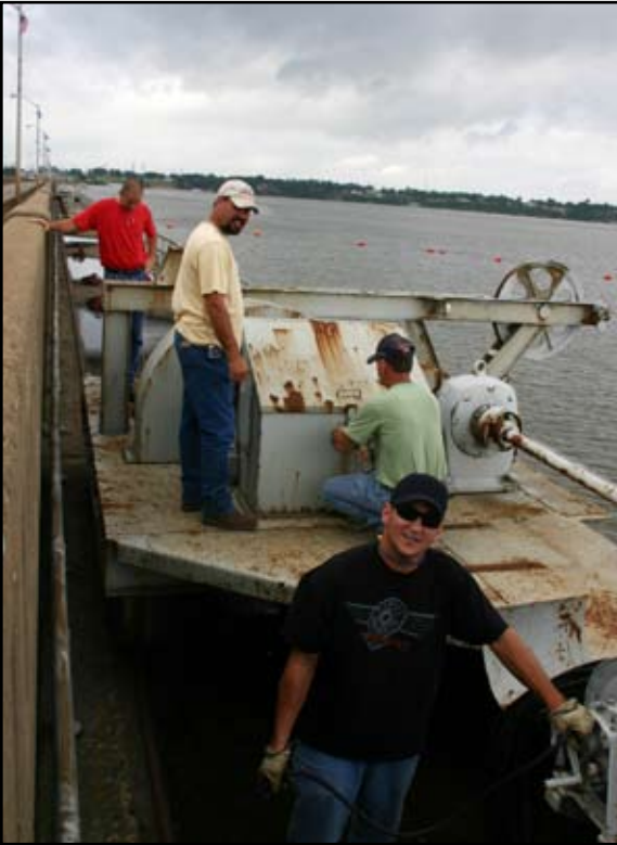
Opening and closing floodgates on the dam is one of the duties of the Pensacola crew.
