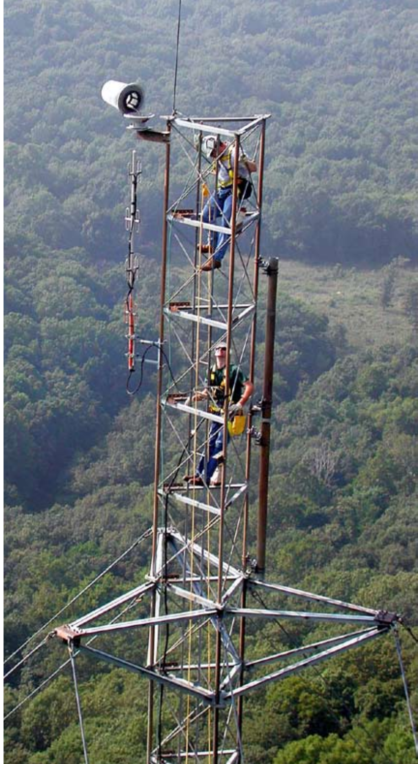
The highest levels of communication... GRDA Communications employees Jimmy Wheeler and Kevin Wheeler (no relation) make their way up a GRDA repeater tower site to do maintenance on the tower light. The Wheelers are just two of the many employees within the GRDA IT Department responsible for maintaining the many information delivery systems vital to GRDA’s daily operations.
