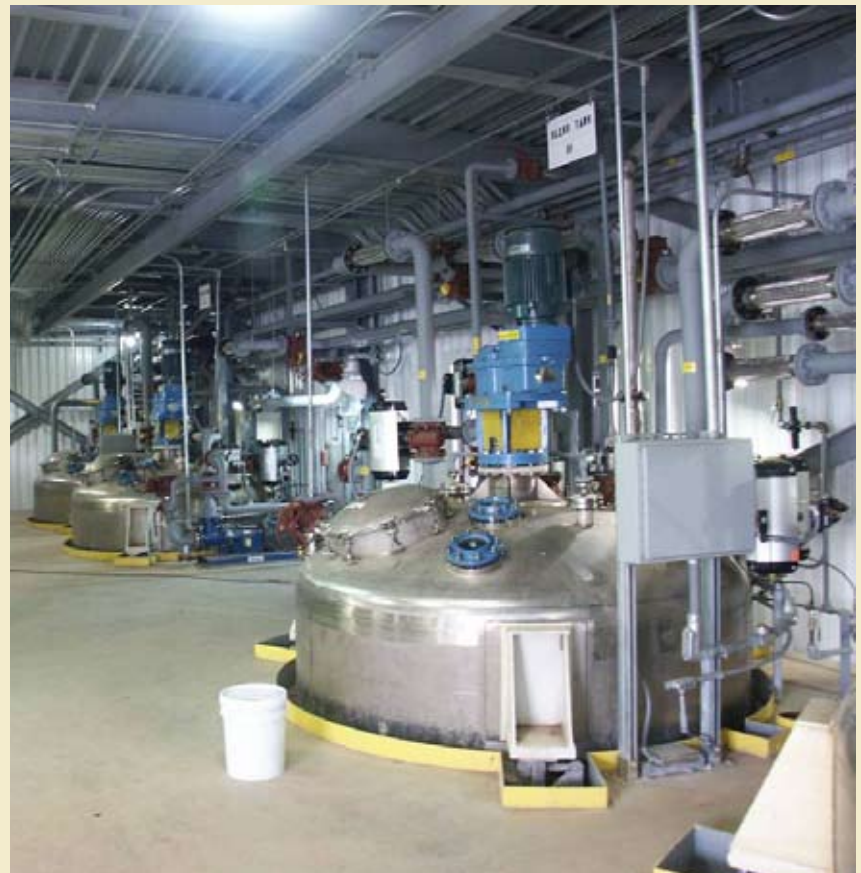
Interplastic Blend Tanks at the MAIP facility.
