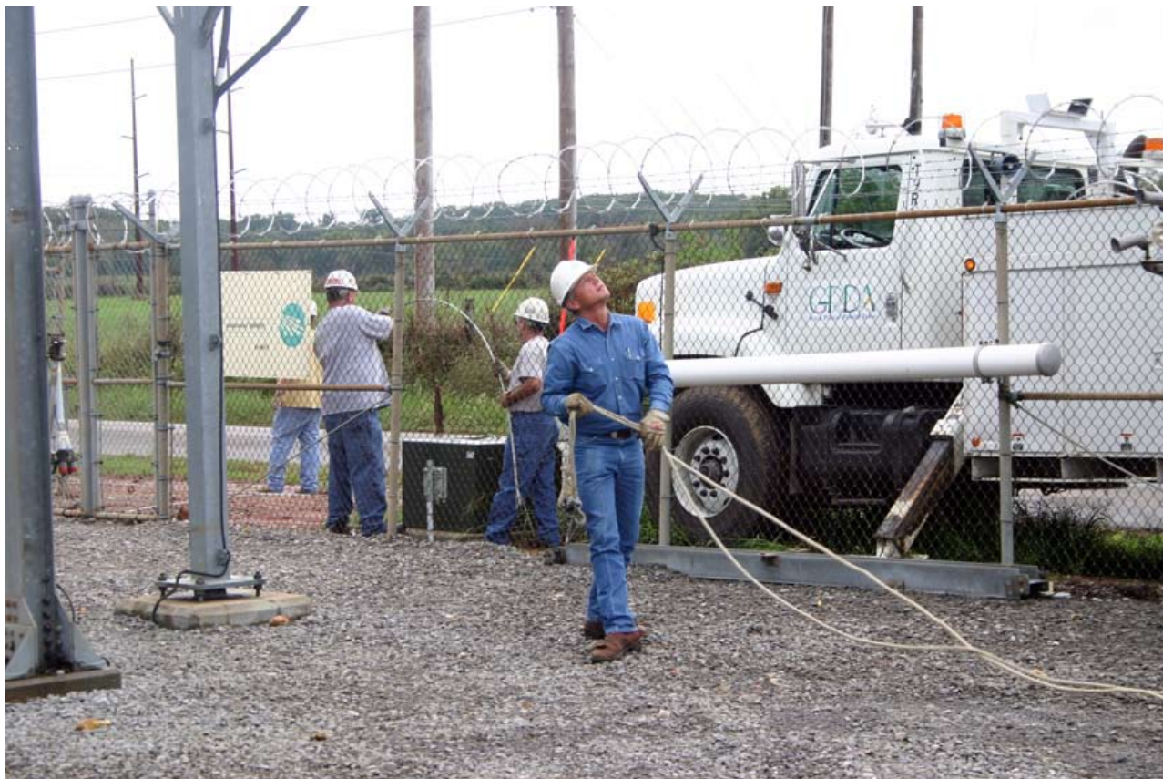
GRDA Lineman Dave Hefner works inside a substation near the GRDA municipal customer community of Stilwell. Fitch Ratings cited new long-term agreements between GRDA and its municipal customers as one of the reasons it has upgraded the utility's credit rating.
