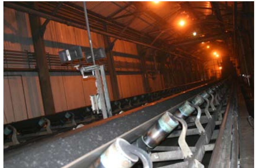
Coal moves along a conveyor, into the main plant.
