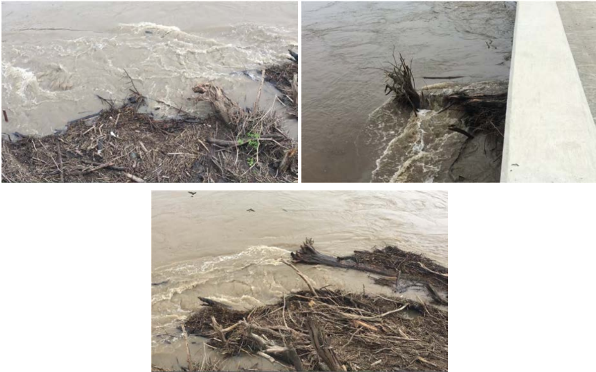
Figure 73 May 2019 Photographs of Debris Trapped on Bridge Piers
