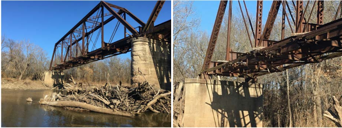
December 2019 Photographs of Debris Trapped on Bridge Piers
