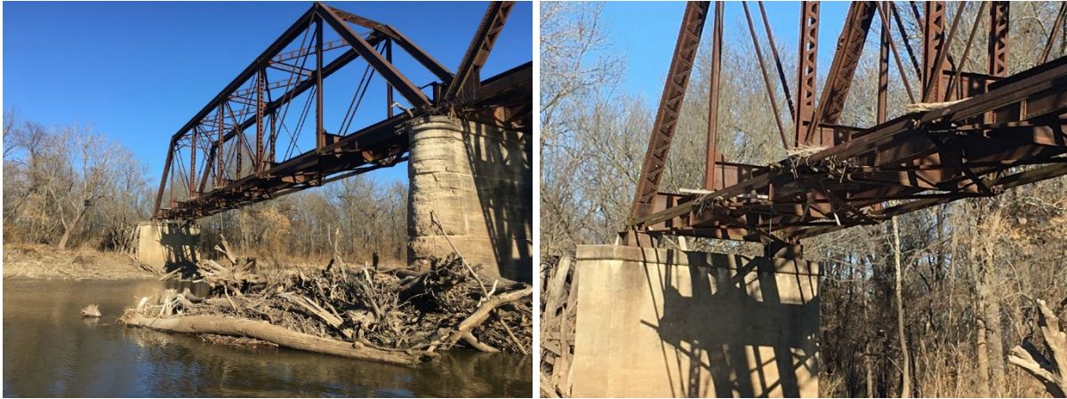
Figure 74 December 2019 Photographs of Debris Trapped on Bridge Piers
