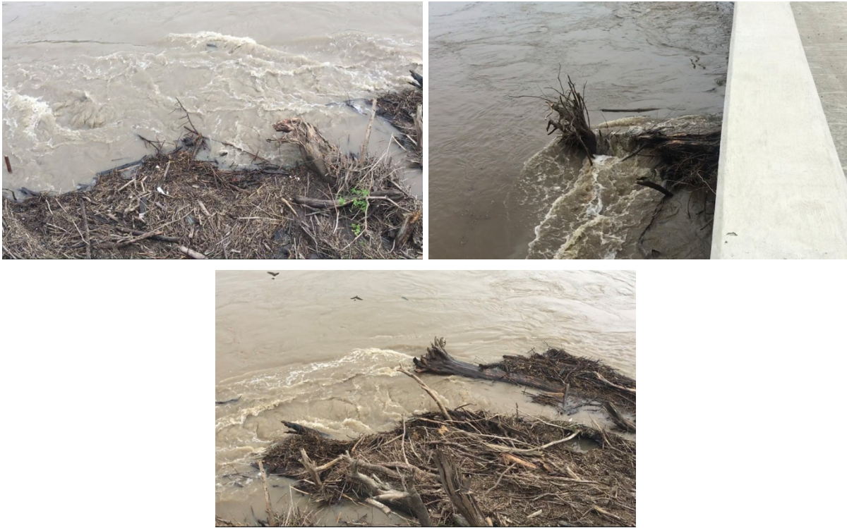
Figure 71 May 2019 Photographs of Debris Trapped on Bridge Piers
