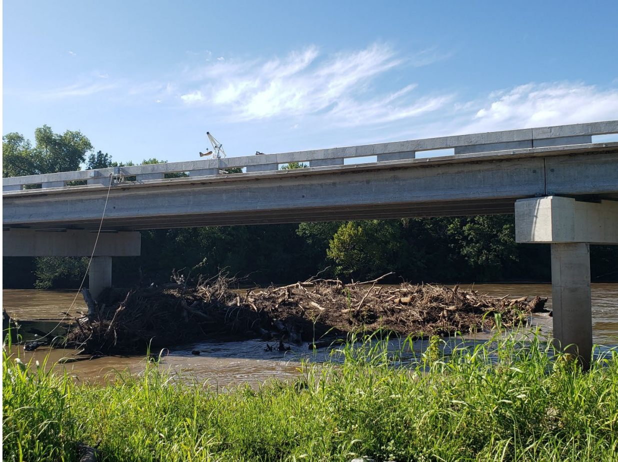
Figure 6 Photo of blockage taken in August 2019. Debris pile remains in place and has grown since photo was taken.
