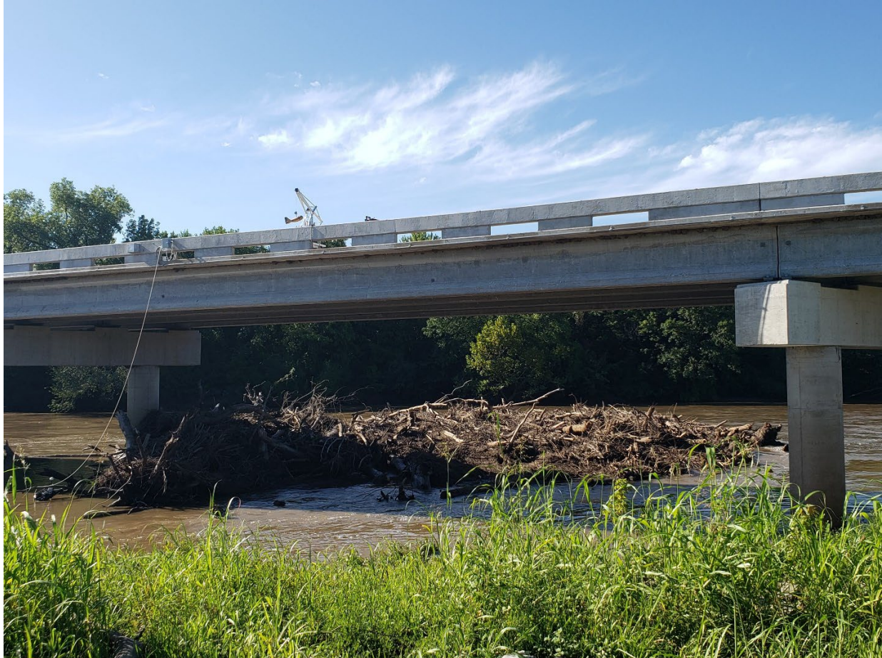
Figure 6 Photo of blockage taken in August 2019. Debris pile remains in place and has grown since photo was taken.
