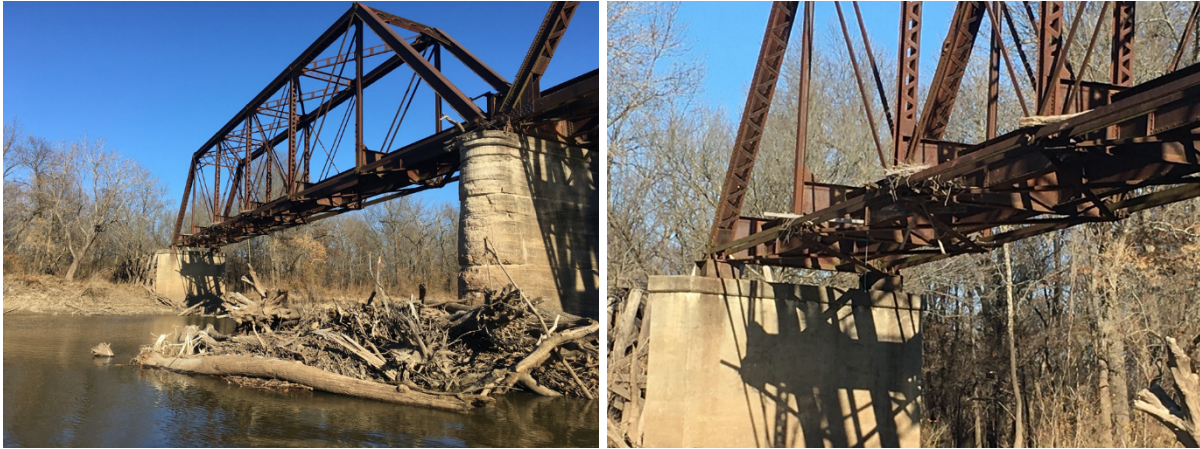
Figure 72 December 2019 Photographs of Debris Trapped on Bridge Piers
