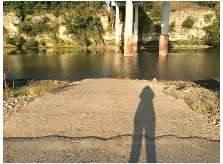
2. Spring River Public Access - September 26, 2020; view west. Low water level recorded at 742.2 feet.
